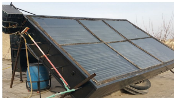
Fig. 1. Overview of the installed flat plate solar collector.
