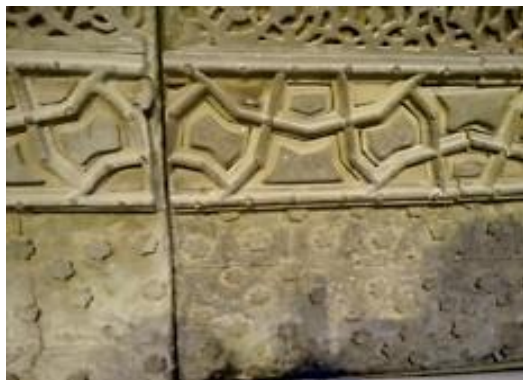
Fig.20. Erosion in the lower parts of the plaques
