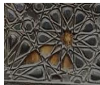
Fig.17.Missing decorative units on the right wing of the planks
